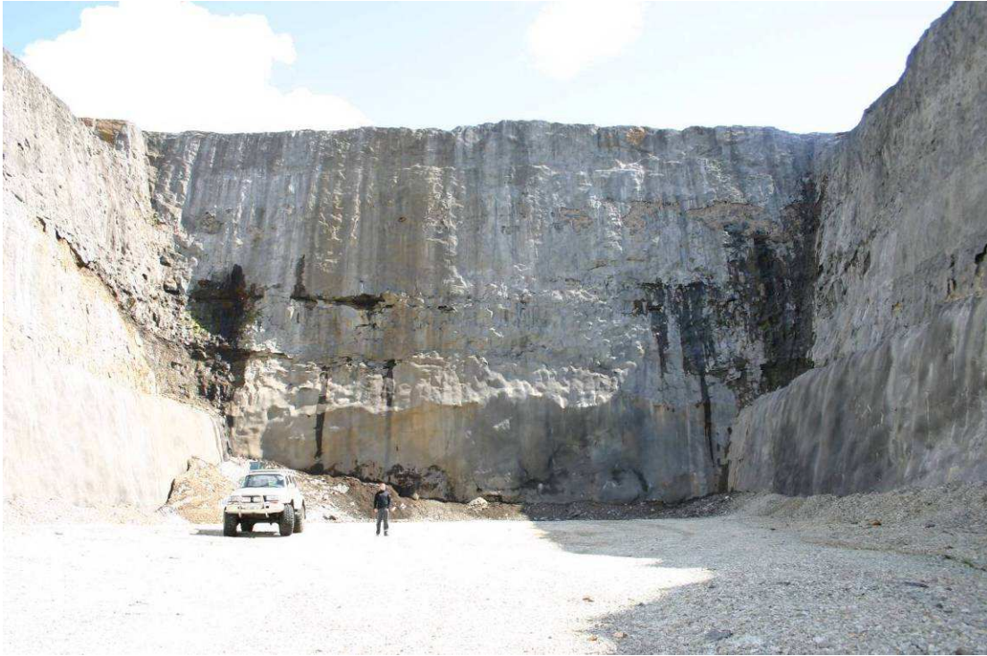
Figure 9-6. Excavation at Búðarháls Power Station foundation, sprayed concrete on walls [Gunnarsson photo, 2009].
